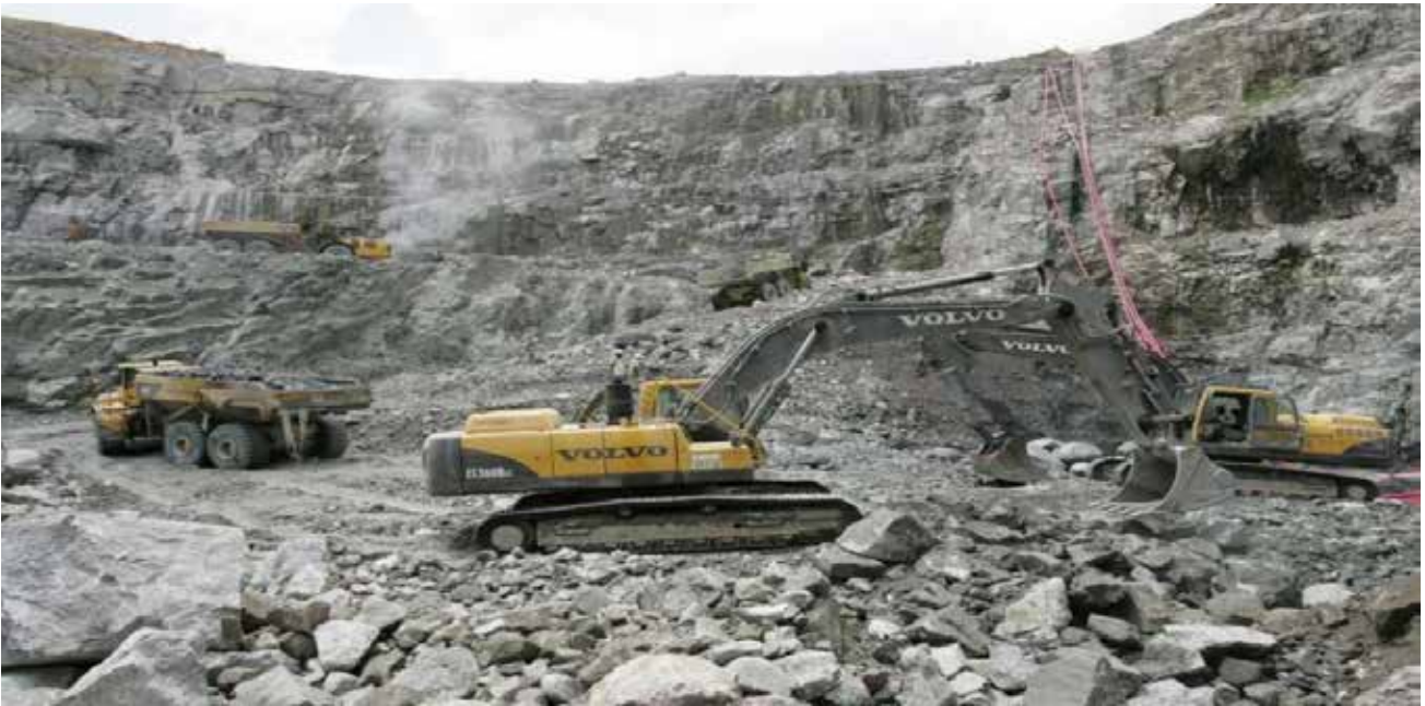
FIGURE 1: Destroying our valuable mountains for the quarrying of aggregate
